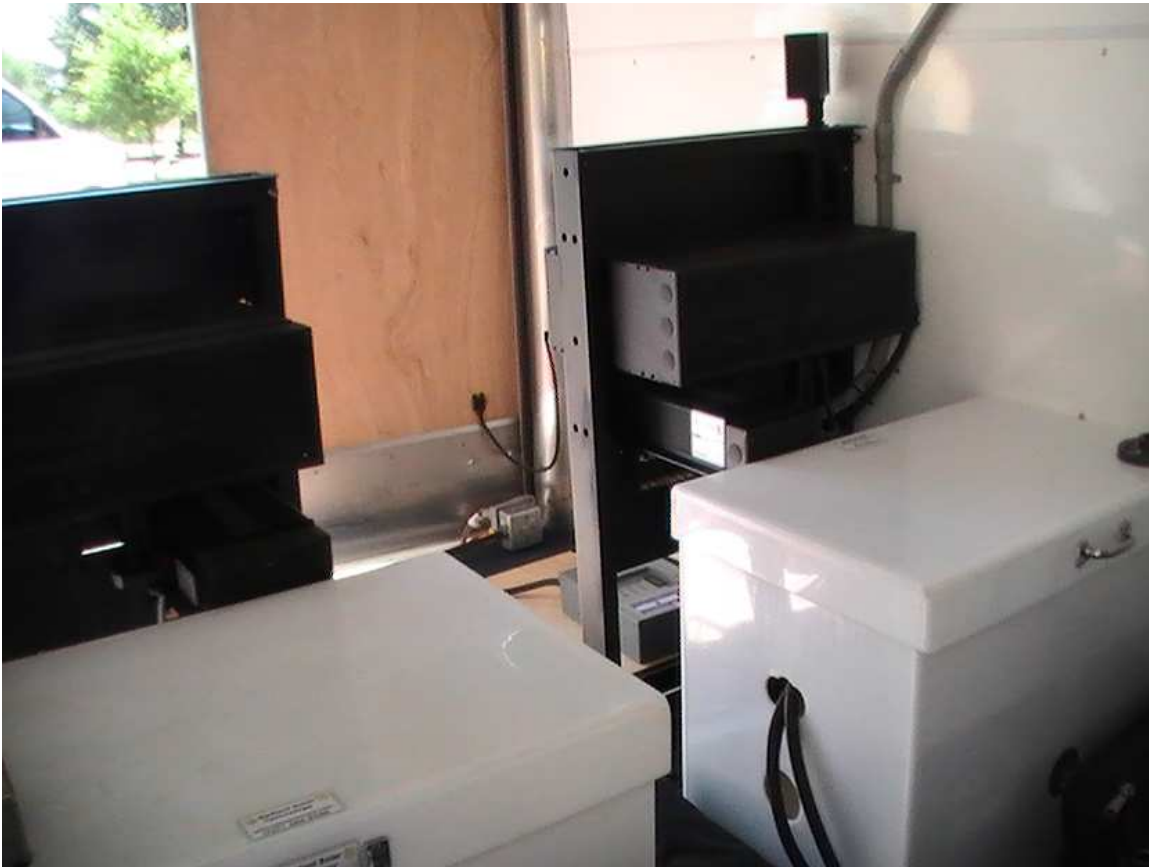
Solar Shuttle Interior – View from Inside Looking to the Rear The Two Large White Battery Enclosures in the Foreground Hold More than 1/2 Ton of Battery.
